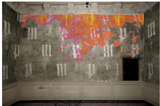
Figure 13: Representation of areas of detachment detected by IRT on room dn west wall © Tedeschi & Cucchi.
