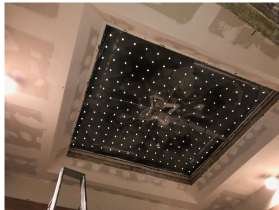
Figure 6: Funicular shell mounted in the opening of the transmission loss facility, with retro reflecting stickers glued on the dome, at the bottom.
