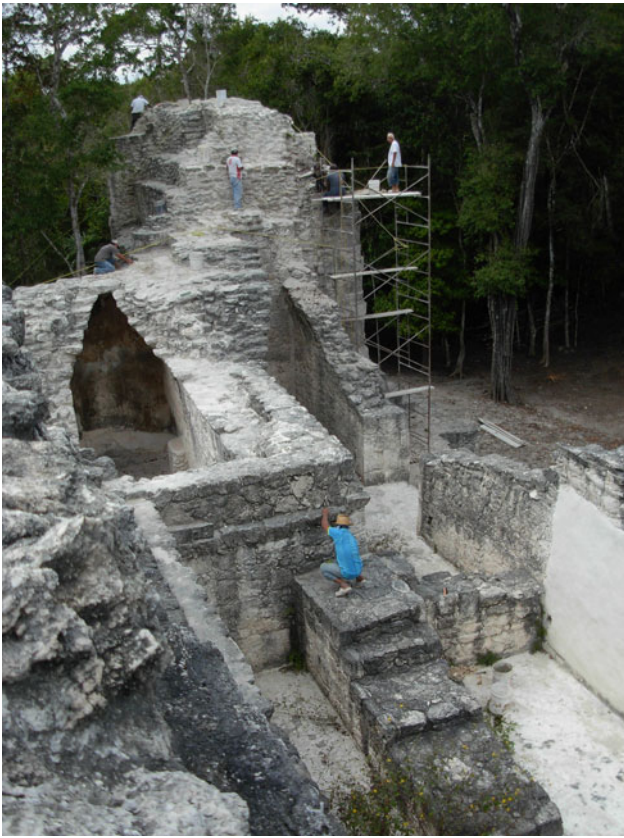
Figure 10. Northwest portion of the final Structure 5N2 building. In the foreground, the worker is on the division wall between Rooms b and c, which leans on the northeast corner of Room g. Photo courtesy of the Río Bec Project.
