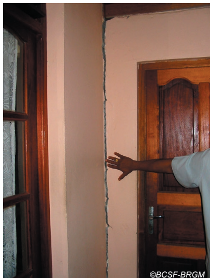
Fig. IV-73. Bouillante - quartier Courbaril - large fissuration.
