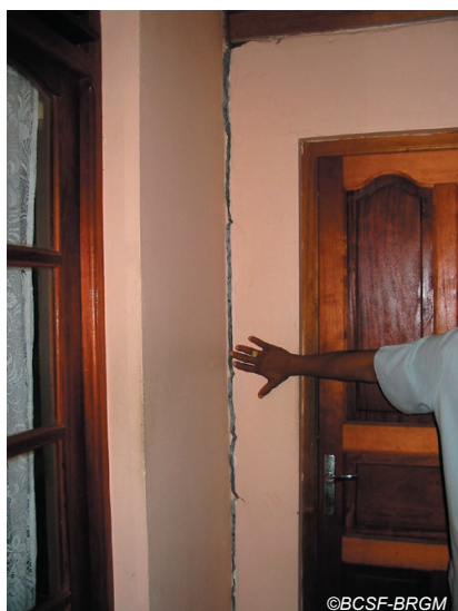
Fig. IV-73. Bouillante - quartier Courbaril - large fissuration.
