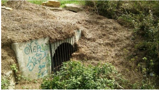
Fig. 6: Vegetation accumulation at one of the underground sections of the channel.
