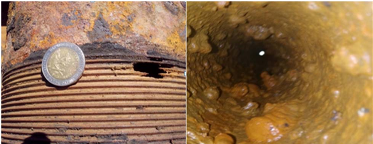
FIGURE 1: Effects of the MIC phenomenon (Left: layer corrosion, Right: biofouling)
