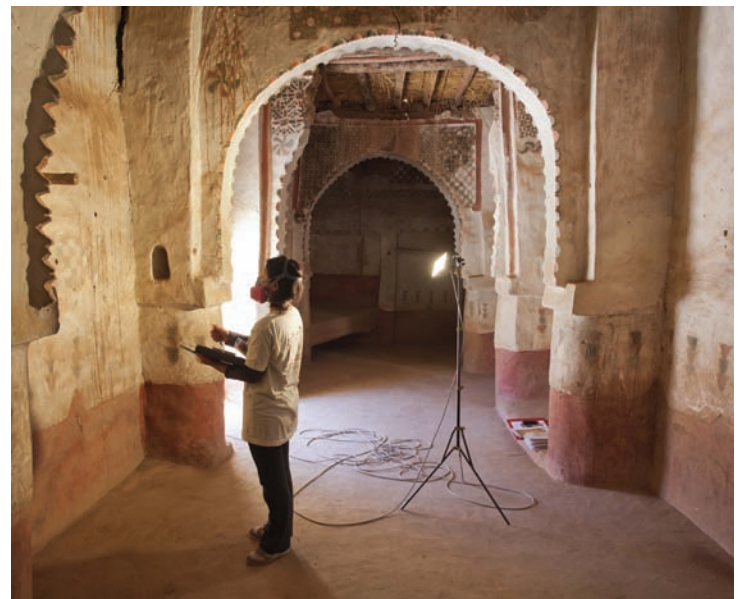
Fig. 8 a graphic condition record illustrating typical deterioration patterns, photo: S. Whittaker
