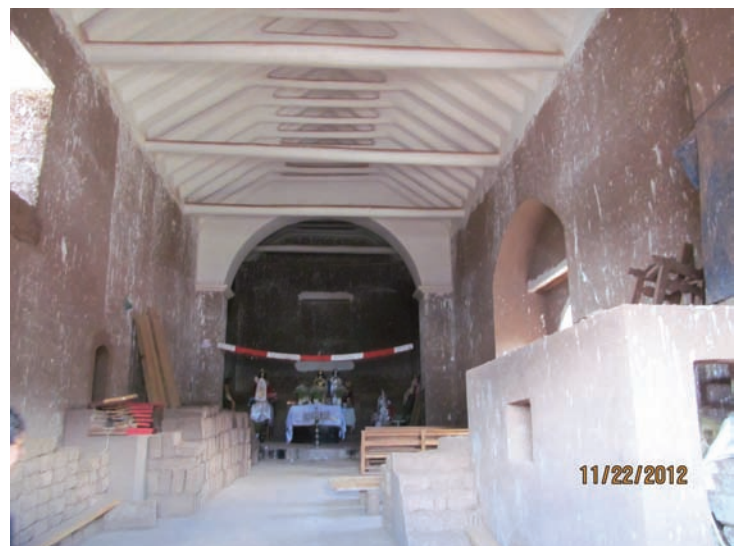
Fig. 1 Interior part of Misca church in Cusco with tie beams, photo: Violeta Paliza
