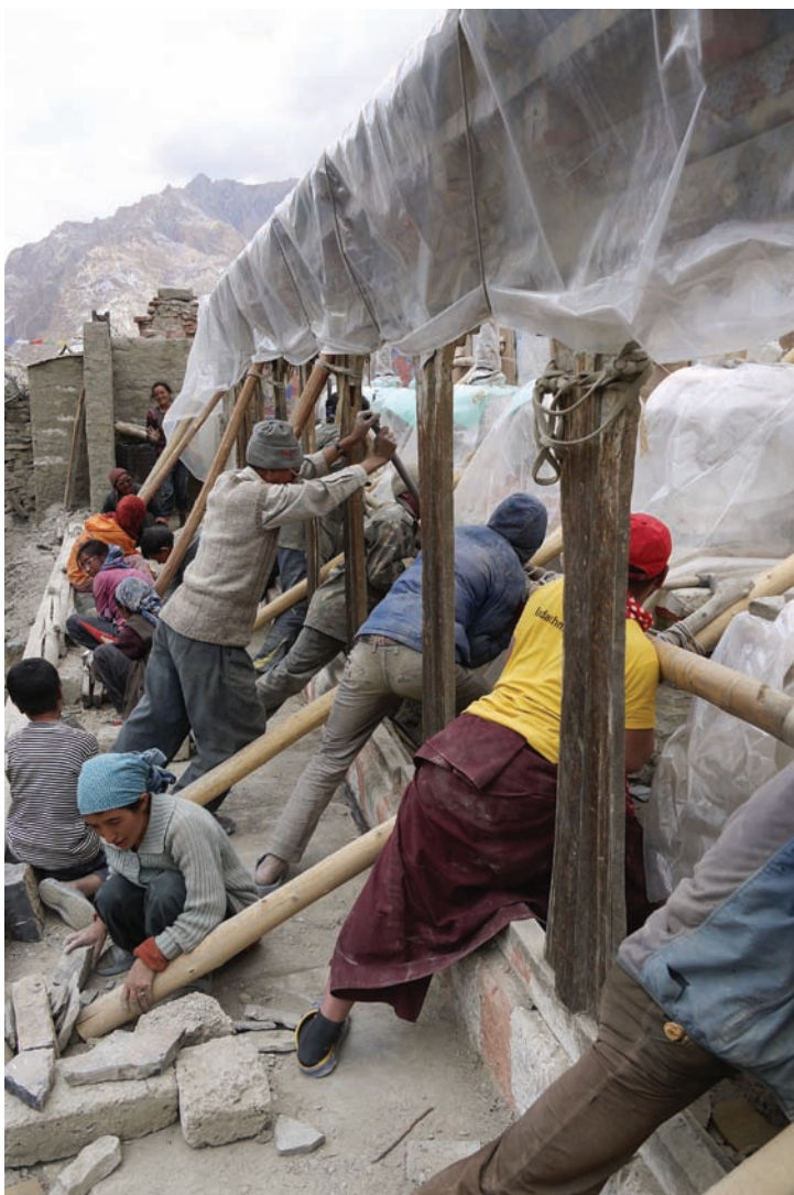
Fig.10 Moving of inclining painted wall back to an upright position, photo: Vets, 2014
