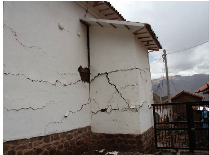
Fig. 5 Structural behavior of a buttress after an earthquake
