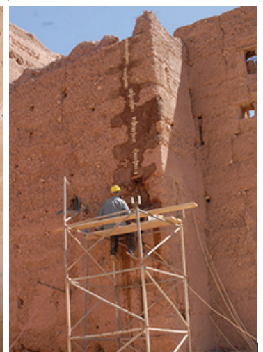
Fig. 10 Conservation works in the Stara, including repairing a structural crack, photo: B. Marcus, 2014
