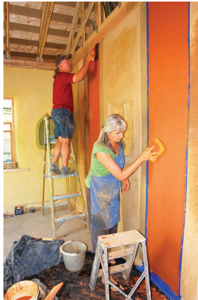
Fig. 1 Bill and Athena Steen plastering a strawbale wall with earth plaster, photo: C. Wanek
