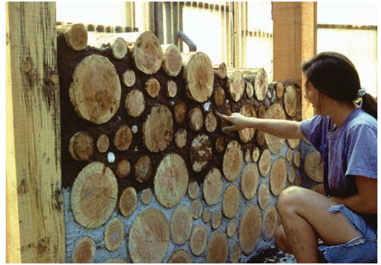
Fig. 7 Using cob as a mortar in a cordwood wall, photo: M. Smith
