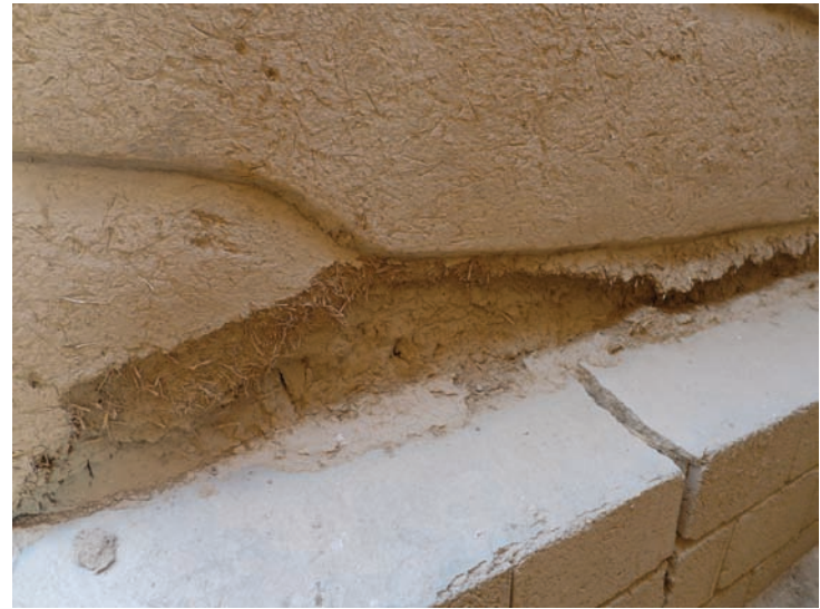
Fig. 4 Concrete-block foundation repair in Najran has caused salt damage
