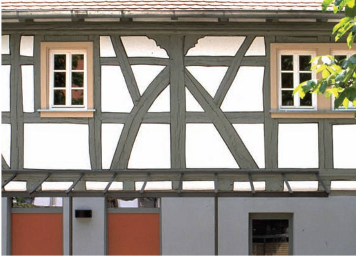
Fig. 6 Restoration with light earth masonry and wattle-and-daub, Mörfelden, Germany, photo: Schauer + Volhard
