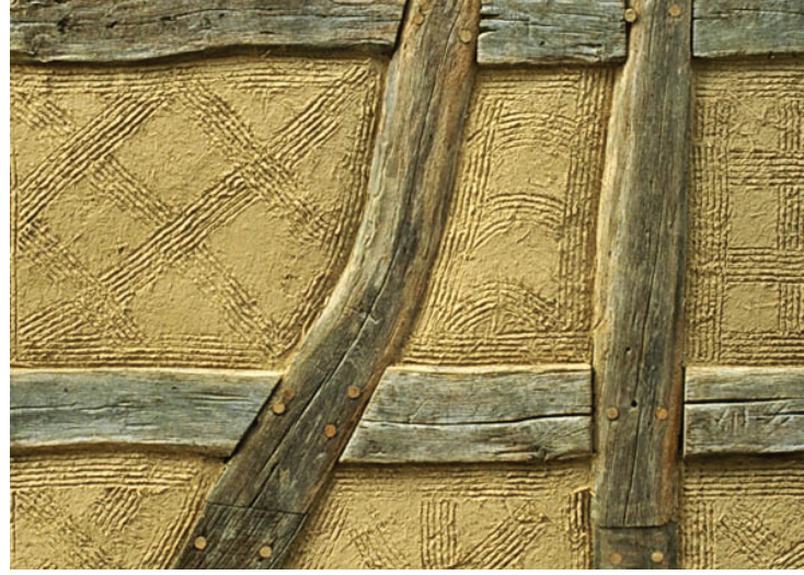
Fig. 7 Straw-clay undercoat plaster with combed ornamentation for the adhesion of plaster, Mörfelden
