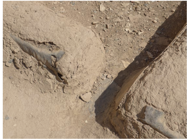
Fig. 10 Compromised rubberized membrane on Al-Emara Palace's roof
