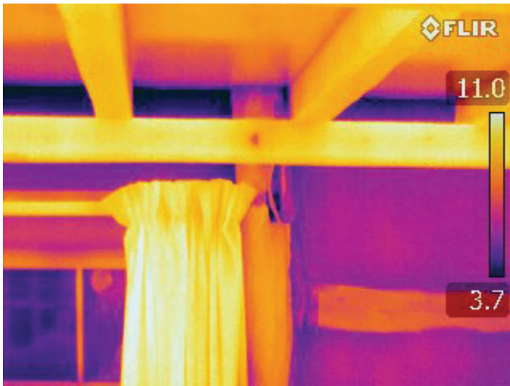
Fig. 3 Internal thermal condition in one surveys M&S building 2015, photo: M. M. Kotakowski
