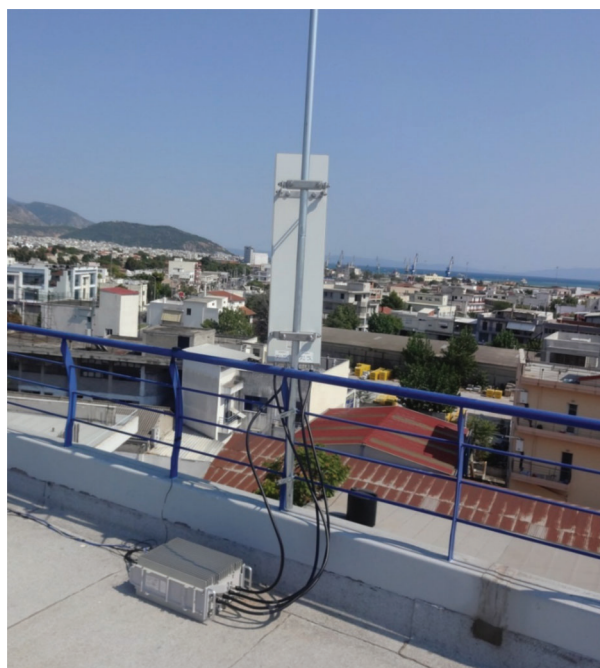
Figure 12.6 WiMAX/LTE Base Station in NITOS testbed.
