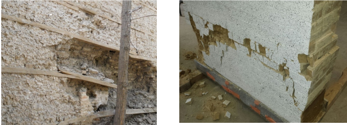
Figure 1. Use of Horizontal timber shear band in Turkey (left) [Photograph copyright: A. Caimi] and prevention of in-plane shear crack propagation with the use of shear band (right) [Photograph copyright: Florent Vieux-Champagne]
