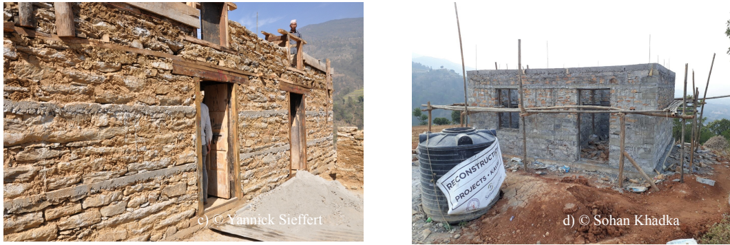
Figure 2. a) Use of stone as a shear band, b) Timber shear band in brick masonry, c) Use of concrete and timber shear band in clay mortar masonry and d) Concrete shear band in cement mortar masonry building
