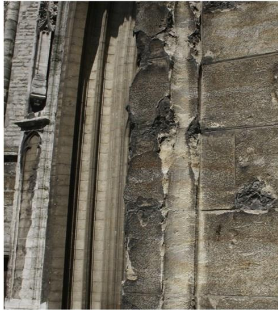
Fig. 3. Weathering pattern of the Lede stone at the Saint Bavo's Cathedral (Ghent, Belgium), where the black gypsum crust is visible and is peeling-off.
