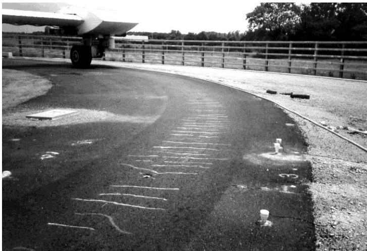
Figure 6. Transversal cracking observed on structure 9.
