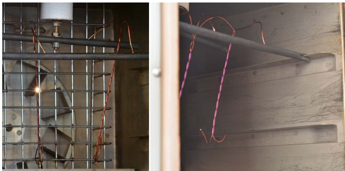
Fig. 3: Testing twisted pairs' installation and appearance of corona effect (purple light on the twists)
