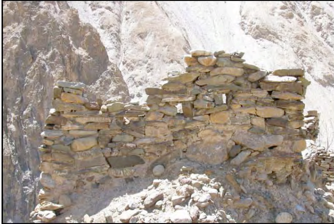
Fig. 40: Multi-colored cobble masonry: stones are mainly cobbles and are of several colors, the most noticeable and characteristic being green. The stones come from fluvio- glacial sediments, visible at various locations in the valley. Tower of Thangring, the wall is about 1 m high. [credits: Devers 2009]
