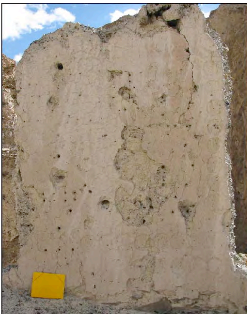
Fig. 16: Chalak: wall with the contiguous rows of circles on the left and on the bottom. The yellow folder is 24x31 cm. Wall made of mud-bricks (26x20x10 cm). Circles are 14 cm in diameter. Picture taken from the south. [credits: Devers 2009]
