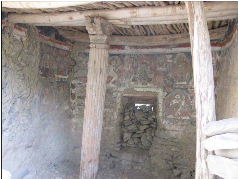
Fig. 25: Markha: interior of the chorten viewed from the collapsed wall. The original door is now closed with piled stones (background). The fluted column with the engraved capital is in the middle (see fig.26). The murals are probably from the 14th century and the column from the 12th century. [credits: Devers 2009]
