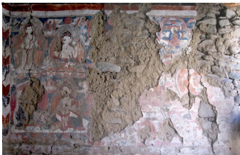
Fig. 9: Left wall. This image is the result of the merging of several pictures – there might be as such a bit of geometrical distortion. (Devers 2009).
