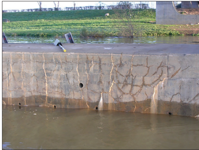
Fig. 1: Cracking of the base of a pylon (Bourgogne bridge: crack width >0.3 mm)
