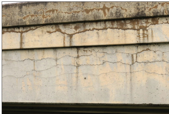
Fig. 2: Longitudinal cracks in the middle of a prestressed precast concrete beam
