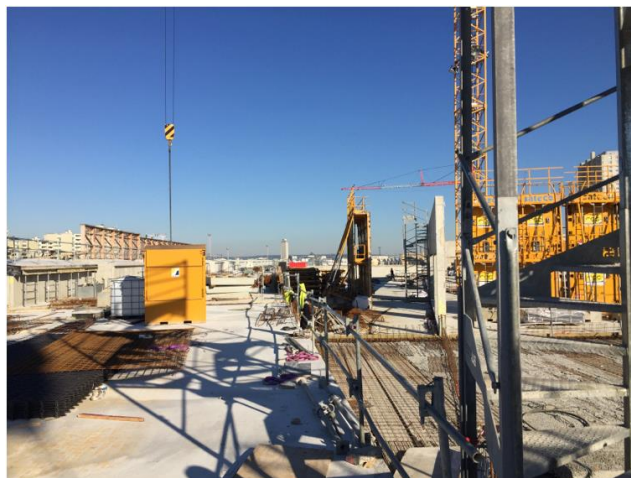
Figure I.10. Chapelle International Sogaris logistics hotel building site, October 2016 Source: photo L. Dablanc
