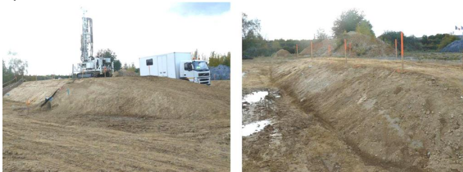
Figure 7. View of the experimental dry dikes built at the Rouen Experimentation and Research Center: on left the lime treated dike and on right the untreated dike
