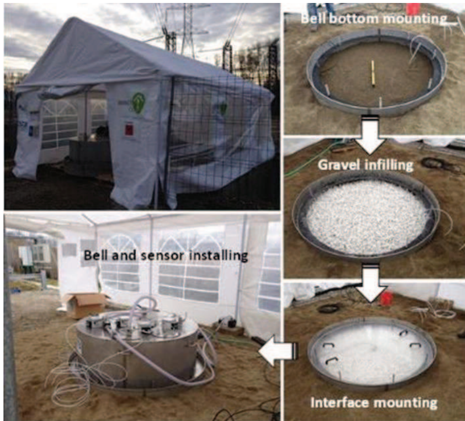
Figure 1 - View of the experimental set-up in the PISCO 2 facilities at Ponferrada. The sequence of pictures on right represents the installation of components.
