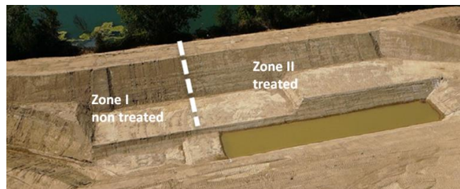
Figure 4. The dike before testing: non treated on the left side, lime treated on the right side
