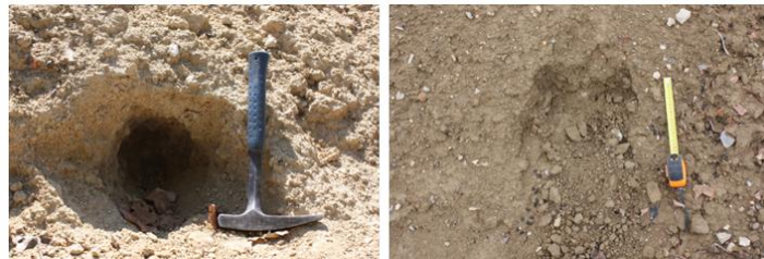
Figure 7. Burrowing animals holes in non treated soil (left) and unsuccessfull attempts in lime treated soil (right)
