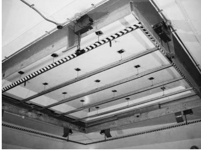
Figure 7. Array of battens suspended from a concrete floor before the installation of the ceiling panel.
