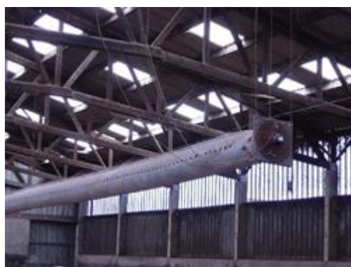
Figure M14.1. Duct for dispersing the tracer gas within a building (source: INRA)
