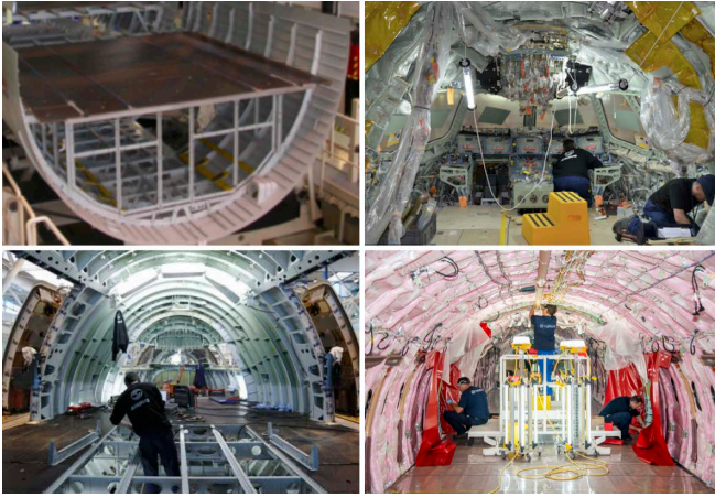
Fig. 1: Example of shop floors and environments (from left to right, top to down): the cargo area, the cockpit, the upper-area in two different phases of the assembly/installation. Notice the postures of the workers. A humanoid is expected to have such accessibility capabilities.
