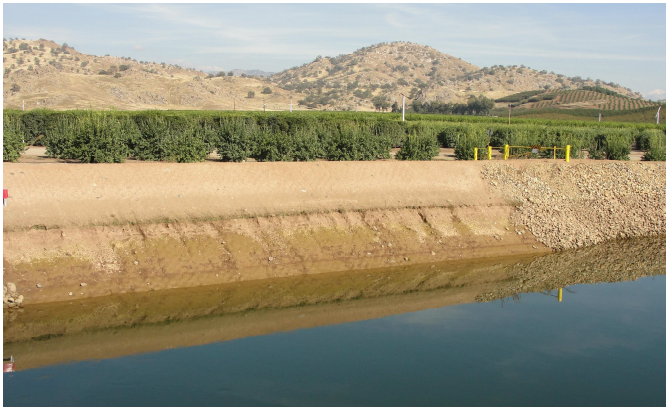
Figure 1: Lime-treated section of the Friant-Kern Canal (taken in November 2010) on the left part; the right part consist of original, untreated slope covered with gravel.
