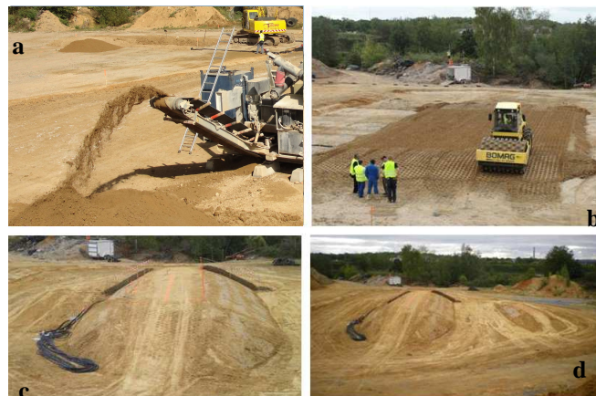
Figure 11: Lime-treated material production (a), application and compaction with a sheepfoot roller (b), global view of the lime-treated dike (c) and of the two dikes (lime-treated and untreated, on the right) (d).
