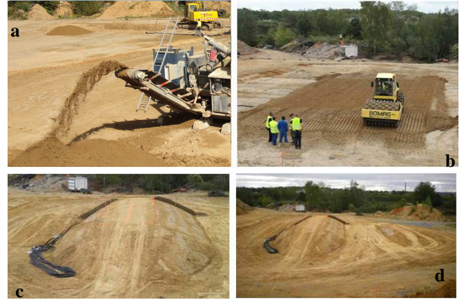
Figure 11: Lime-treated material production (a), application and compaction with a sheepfoot roller (b), global view of the lime-treated dike (c) and of the two dikes (lime-treated and untreated, on the right) (d).
