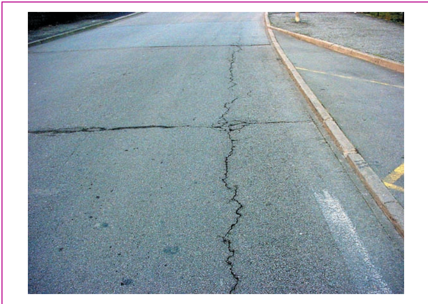
□ Figure 1 Example of a semi-rigid, cracked pavement
