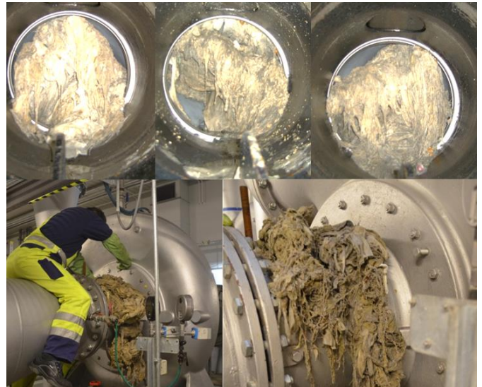
Figure 7. Fibre accumulation in front of the impeller and pump cleaning at the observed pumping station [8]
