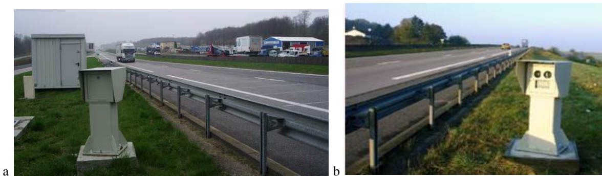
Fig. 1. Standard WIM station in France: (a) WIM sensors in the pavement; (b) cameras in the road side cabinet.
