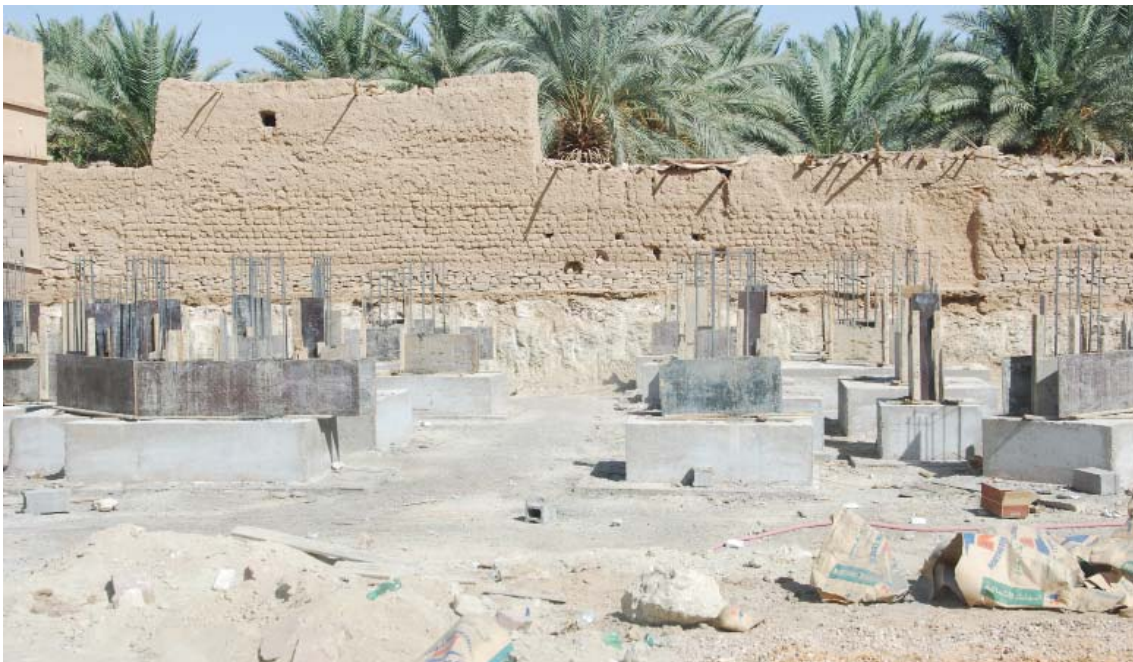
Fig. 4. House basement built at the location of the as-Sunamiyat necropolis excavated by the Saudi Team in 1985-1986
