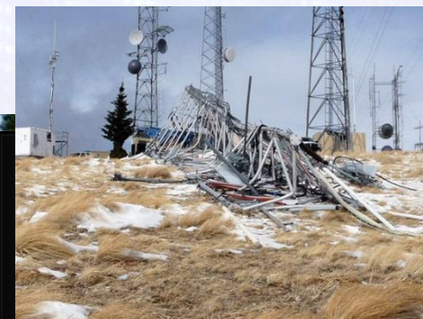
High winds win over tower's ability to brace them December 18, 2009 - Winds estimated to be in excess of 100 mph on December 8 were credited with toppling this 143-foot tall self supporting tower on top of Buck Mountain in Ruidoso, N. Mex. The structure is owned by White Mountain Communications of Roswell.
