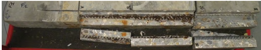
Fig. 4 Post-mortem analysis of the RC sample where corroded and non corroded areas can be observed
