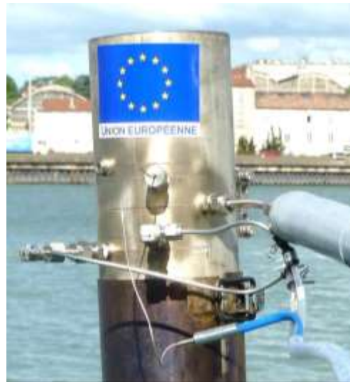
Figure 2: Pitot tube and exhaust gas sampling adapted to the propulsion engine funnel (passenger vessel)
