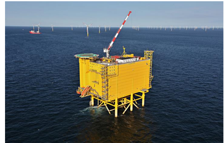
Dolwin wind farm and HVDC converter (800 MW). Document ABB
