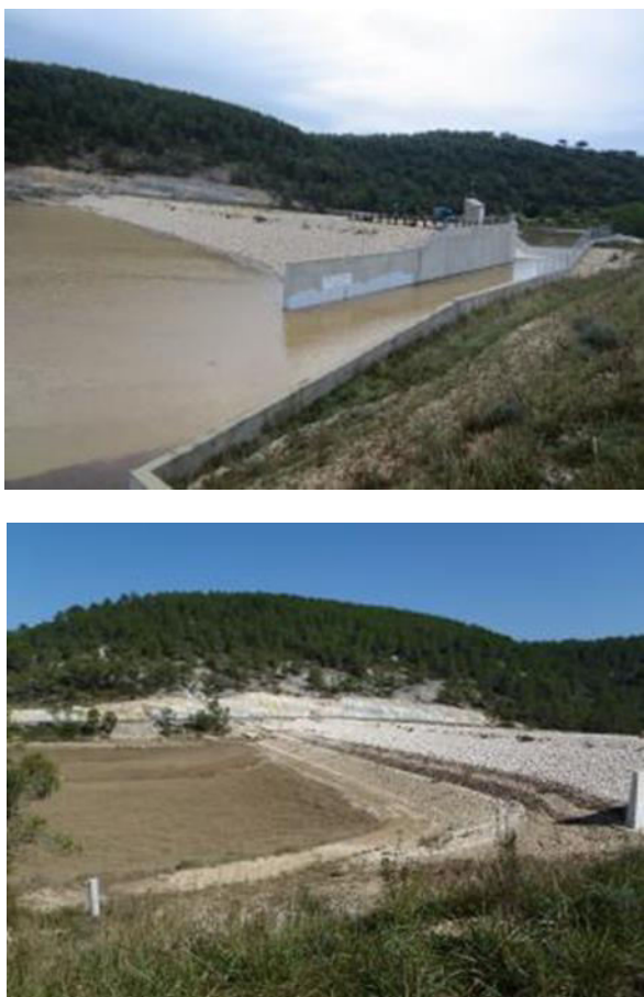
Figure 12. Dam during one of the flood events: during the event (top) / after it has drained (bottom).
