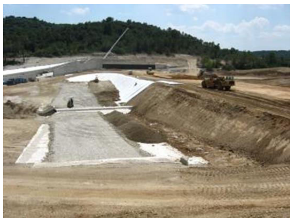
Figure 11. Dam construction site: view of the zoned shell, the bottom sluice, the drainage geotextile, the waterproof core, and the flood gate.
