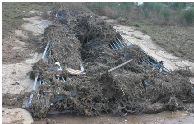
Figure 3. Example of bottom outlet fence collapse.
