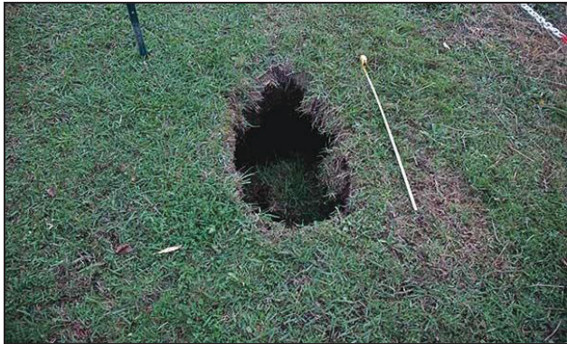
Figure 14. Sinkhole induced by stump decomposition and generating risk of internal erosion (Source: PM)
