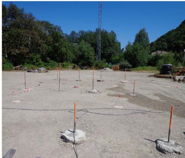
FIG. 8. Photo of a soil reinforced with columns of concrete 0.4m in diameter and 15m in depth (Courtesy of M enard).
