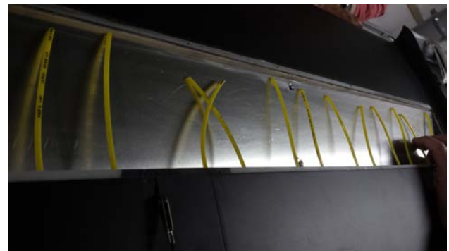
Fig. 14 – View of cooling system
