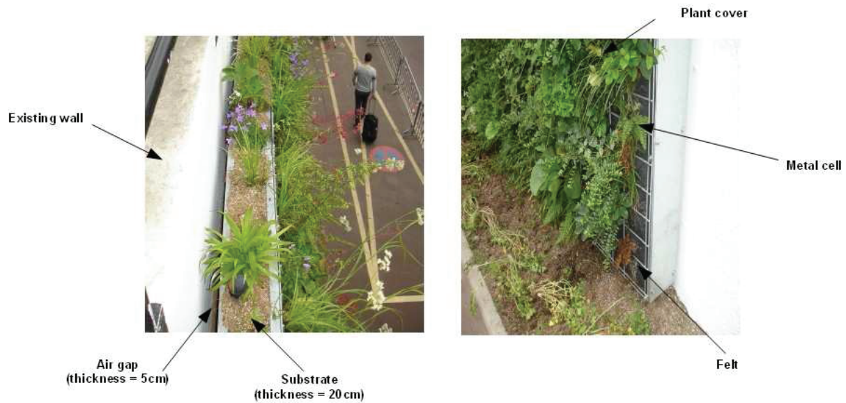
Figure 3 - top view (left) and side view (right) of the green wall
