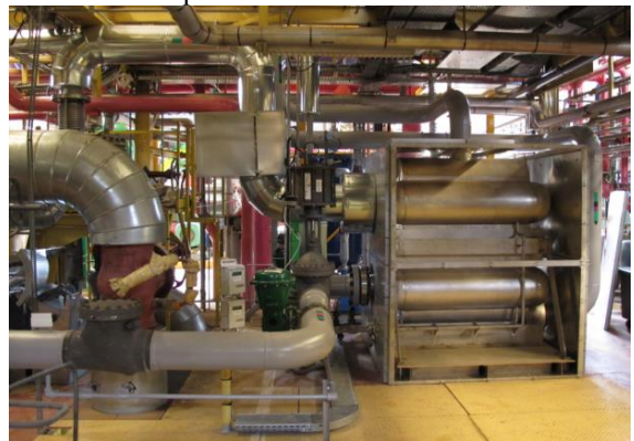
E30 heat exchanger - General Services
