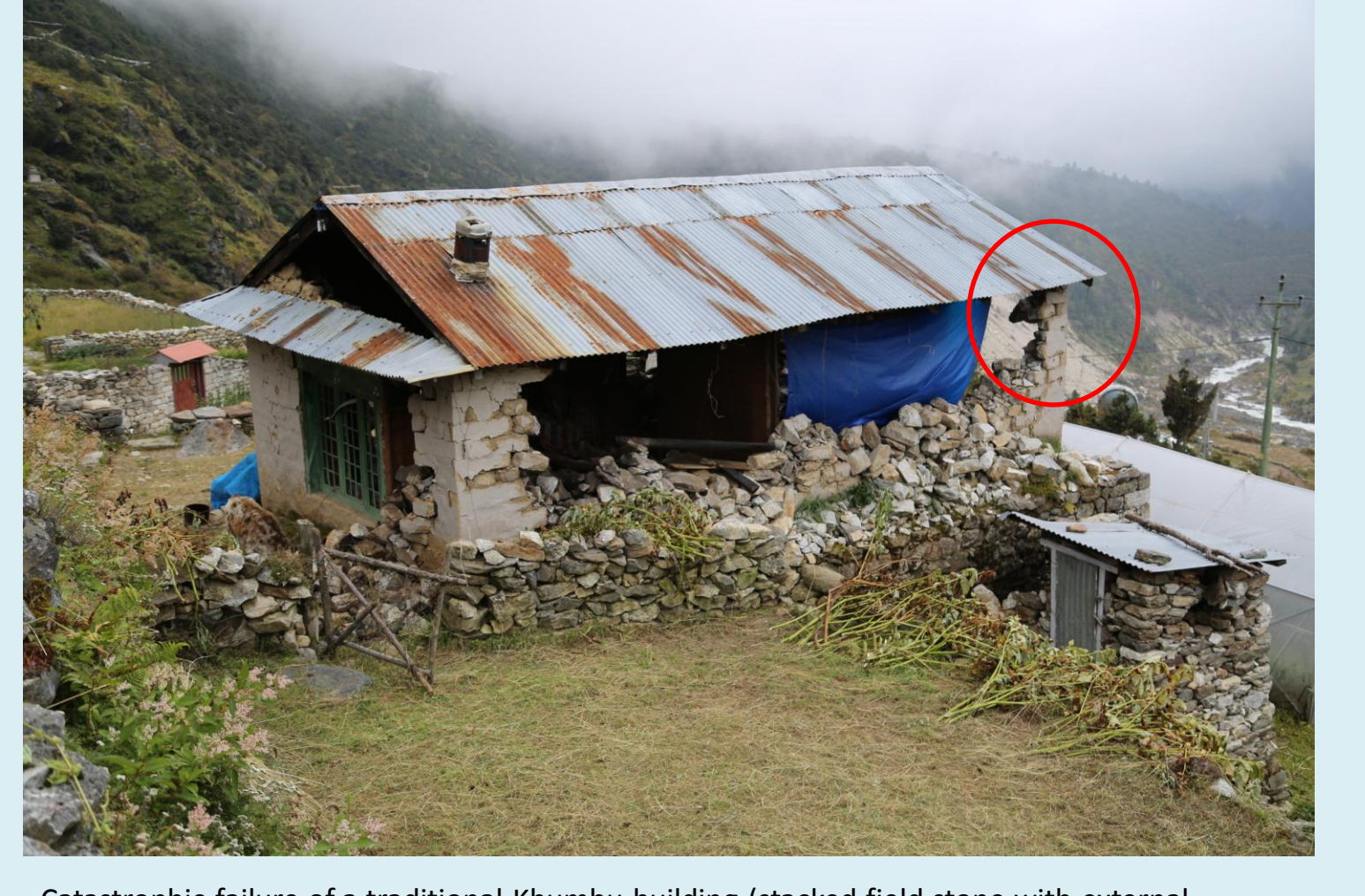
Catastrophic failure of a traditional Khumbu building (stacked field stone with external plaster) near Thame. The entire structure is on the verge of collapse (red circle). An elderly man lives here with a young yak, residing in a small tent on the opposite side of the building.
