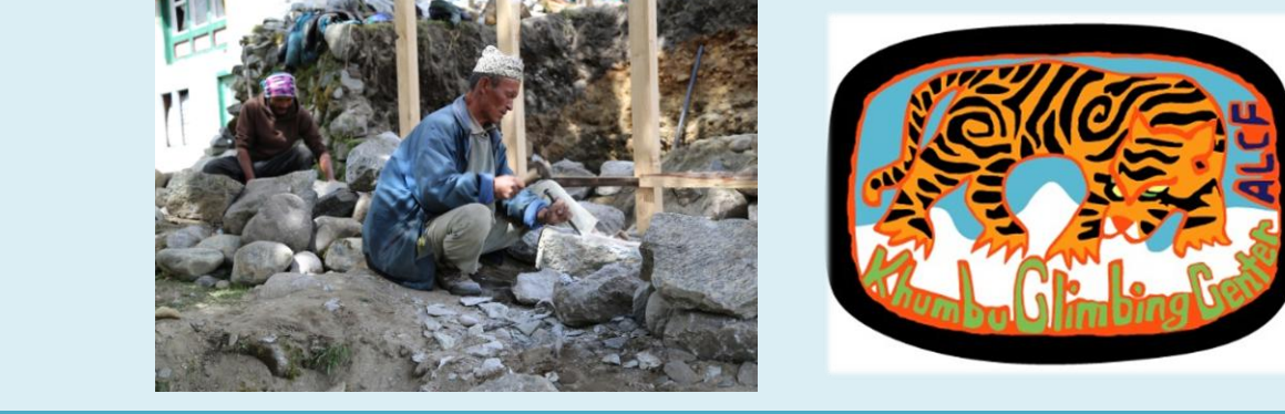
Wire-mesh gabion walls are used in conjunction with expensive steel-frame construction at the Khumbu Climbing Center in the Sherpa village of Phortse, resulting in a reasonably strong structure that withstood seismic shaking in 2015.
