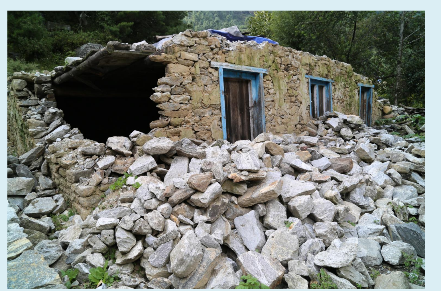
Catastrophic failure of a traditional Khumbu building (stacked field stone – URM).
