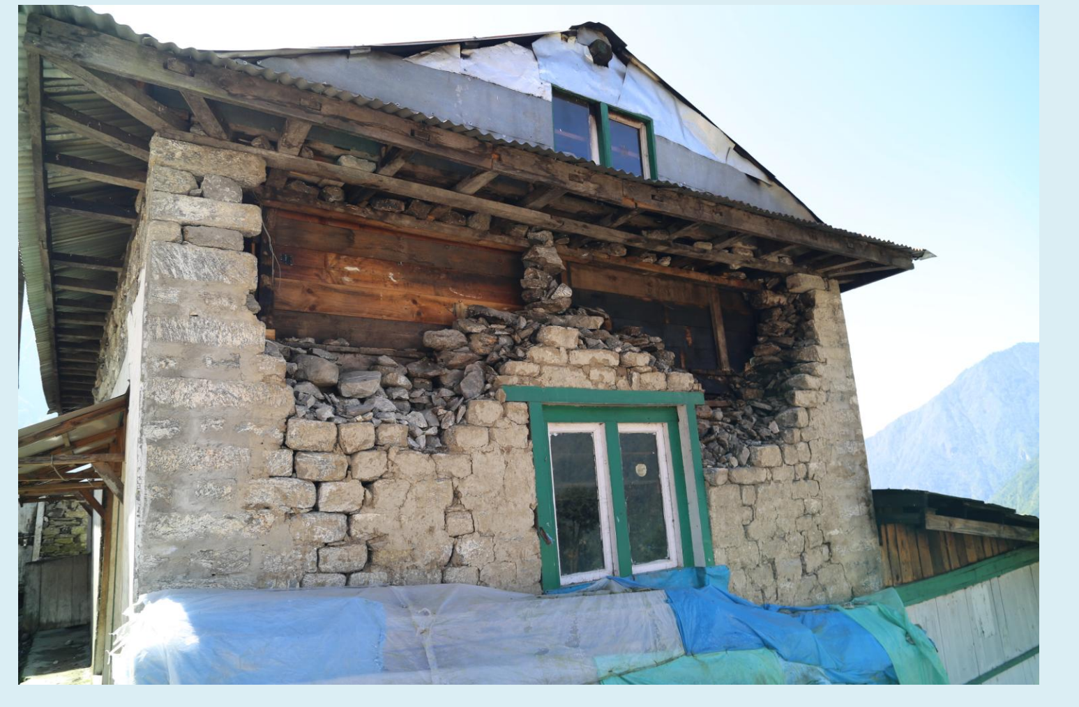
This is typical of structural damage in the Khumbu region. Failure occurred at the top of external rock walls (unreinforced masonry), leaving inside wood paneling exposed but relatively intact. It is likely that this rock wall will be rebuilt in the same style as before the earthquake, due to lack of resources.
