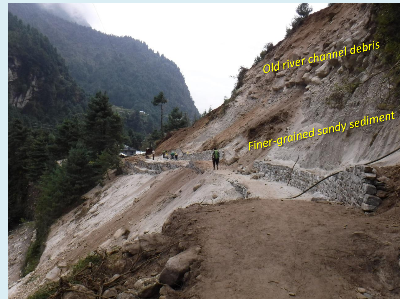
Large earthquake-induced landslide on the west flank of the Dudh Koshi River immediately north of Phakding above the Dudh Koshi River. Workers have started rebuilding the trail across the slide-path (Oct. 2015), despite obvious unstable perched boulders above. The unconsolidated and heterogeneous nature of the coarsely-stratified sediment is obvious.
