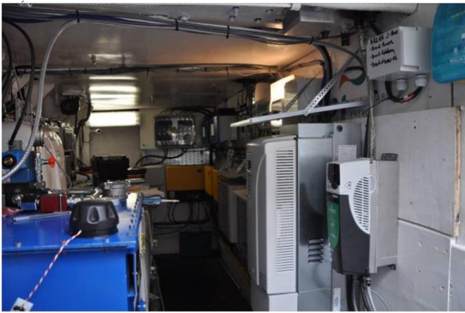
Figure 2 On-board operating and monitoring system
