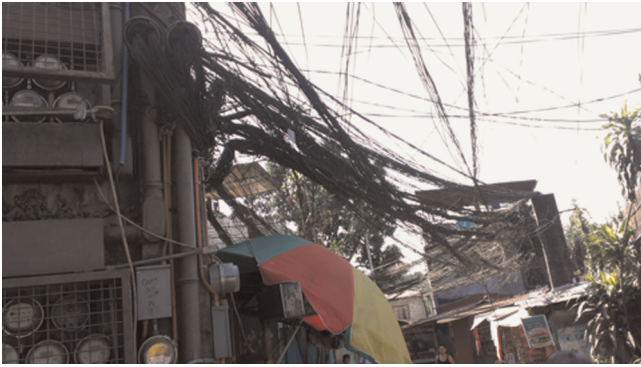
Picture 1. The wires hanging over Pansol in Quezon City, Metro Manila, February 2013.
