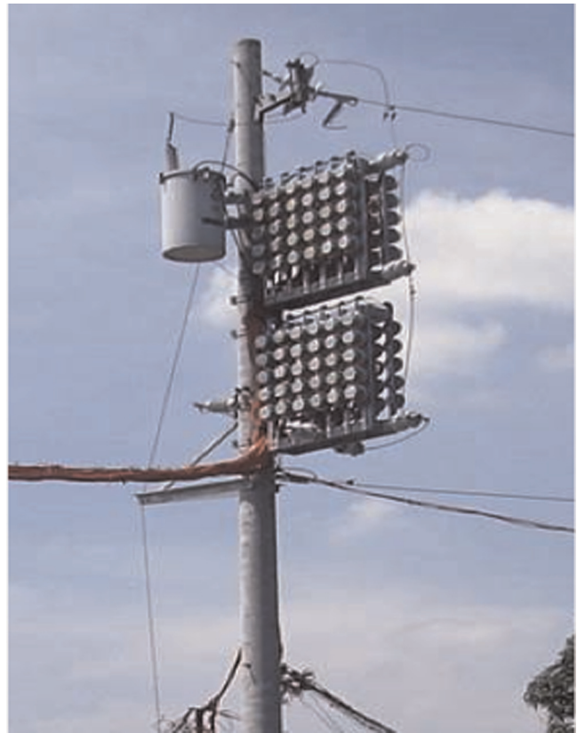
Picture 3. An elevated metering cluster. Source: Meralco, “Delivering electricity to vulnerable communities”, Asian Development Bank Asia Clean Energy Forum, June 19th 2009.
