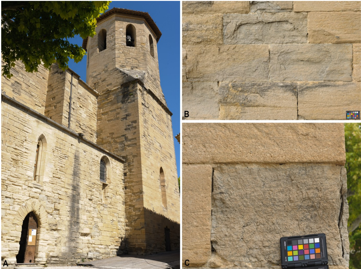
Figure 1. Views of church Saint Maurice of Caromb (14 th century, Vaucluse, France) showing the high degree of spalling decay on the bell tower (A), and the eastern façade (B). The superficial state allows distinguishing a limestone type strongly affected by spalling (grey facies) from one moderately affected (yellow facies). Details highlight the progressive plate formation affecting a grey ashlar viewed from the side (C): the plates vary in thickness and are isolated from the bulk by a fractured zone.
