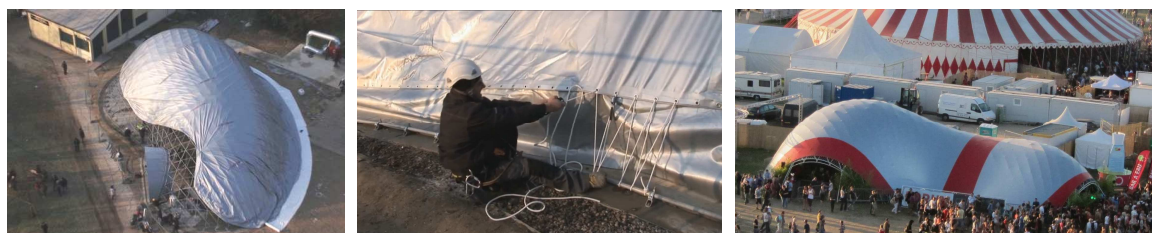
Figure 8: a. Positioning of the PVC coated membrane (Creteil). b. Continuous beam for border during tightening (Creteil). c. Membrane without wrinkle (Solidays gridshell).
