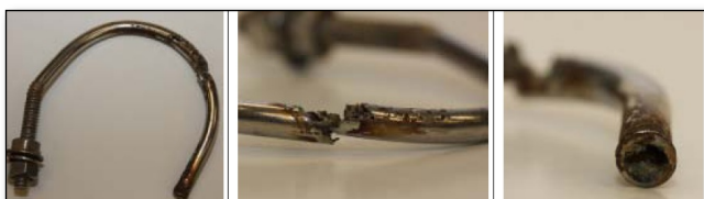
Fig. 10. Stainless steel bracket corrosion [10].
