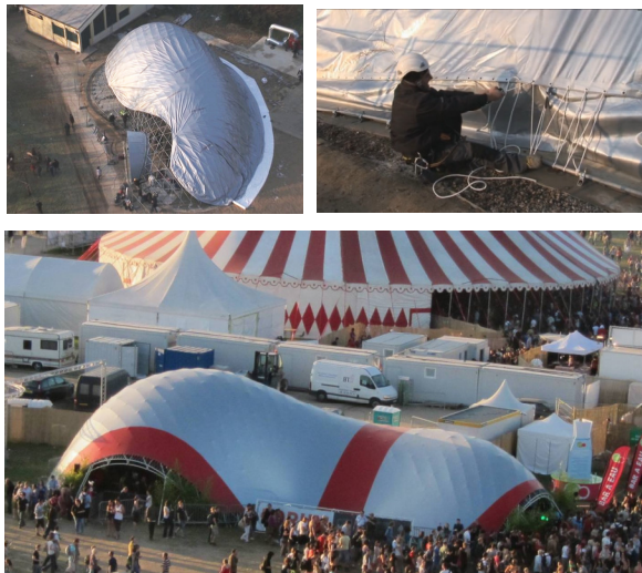
Figure 9: Up: Positioning of the PVC coated membrane (Creteil). Down: Membrane without wrinkle (Solidays gridshell).
