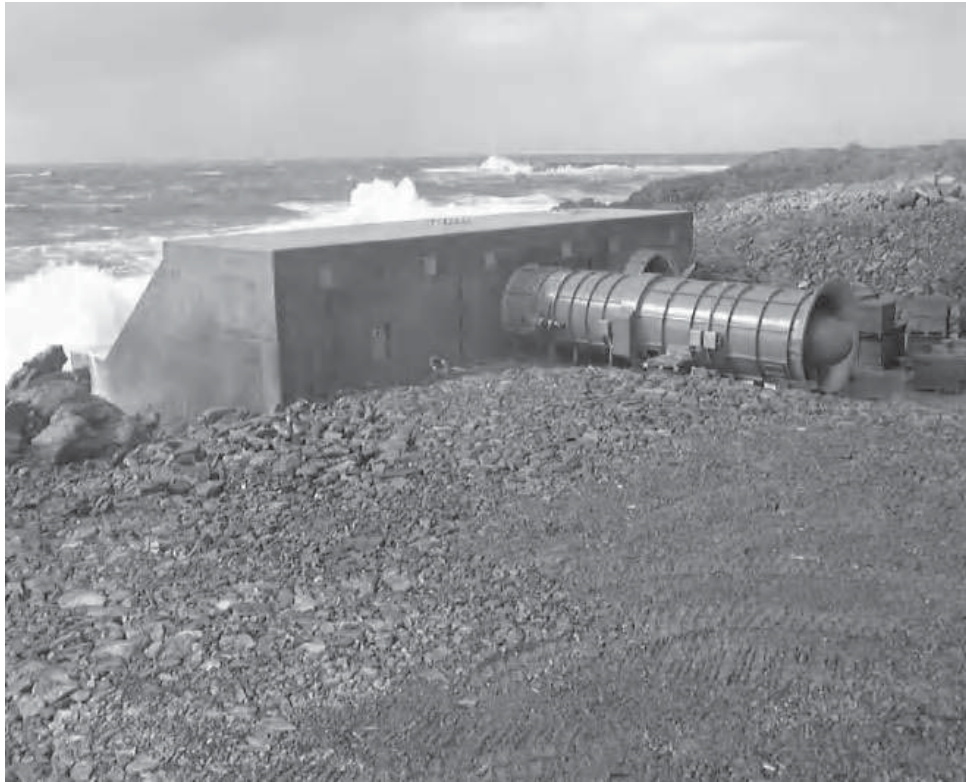
Figure 11.13. LIMPET plant in Scotland [BEL 02]
