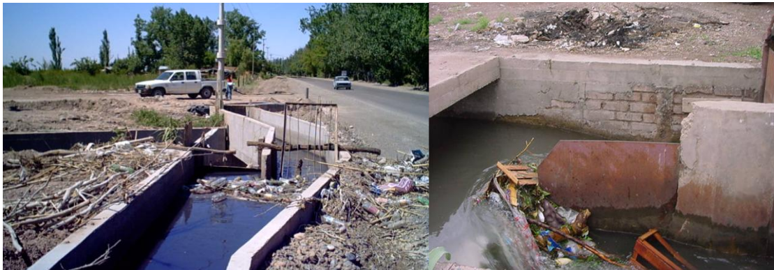
Figure 3: Urban waste in irrigation canals: reduced distribution and application efficiency (Salatino, 2011)
