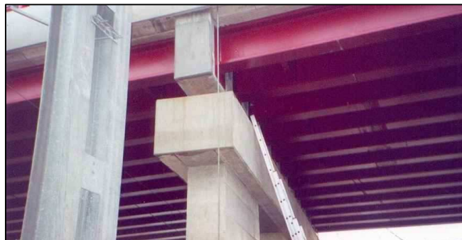
Figure 1 – Beam-to-beam joints with butt-plates connected to a transverse concrete beam in a multi-beam composite bridge.
